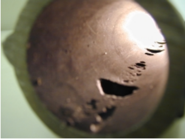
Boiler tube with caustic gouging on the I.D. (end view)
