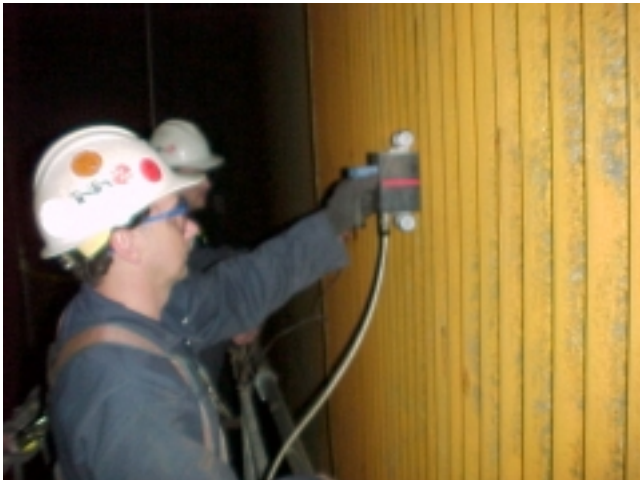
Field service crew performing an inspection of a boiler waterwall.
